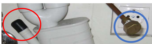
Picture 1. The dishwasher drain hose plug (plastic) and water intake line plug (brass)
